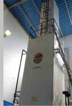
AIR SEPARATION UNIT
